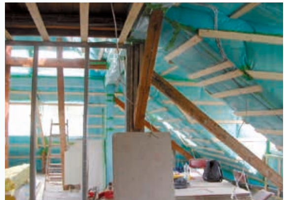
The air barrier is still visible (sheets and wood panels): This is the optimum time for a BlowerDoor measurement.
